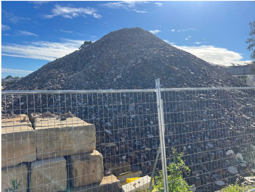
Site Observation: Stockpile of site-won natural material being temporarily stored and used as backfill – in progress. The height of the stockpile was noted as a potential issue, however it is in the process of being reused, and lowered. Refer to Condition D23, OFI-06.
