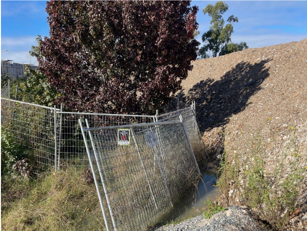
Site Observation: Tree protection with stockpile formed adjacent fence creating water ponding around base of protected tree. Refer to D23, OFI-07.
