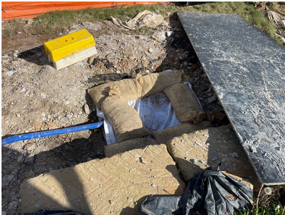
Active dewatering in progress. Water pumped from onsite pool to stormwater in accordance with Council requirements and approvals.
