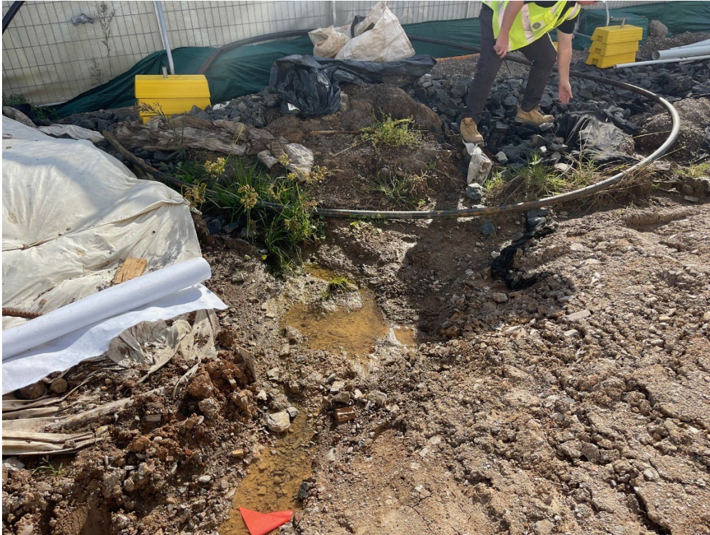
Site Observation: Swale drain requiring maintenance to remove debris. Refer to Condition D26, OFI-08.
