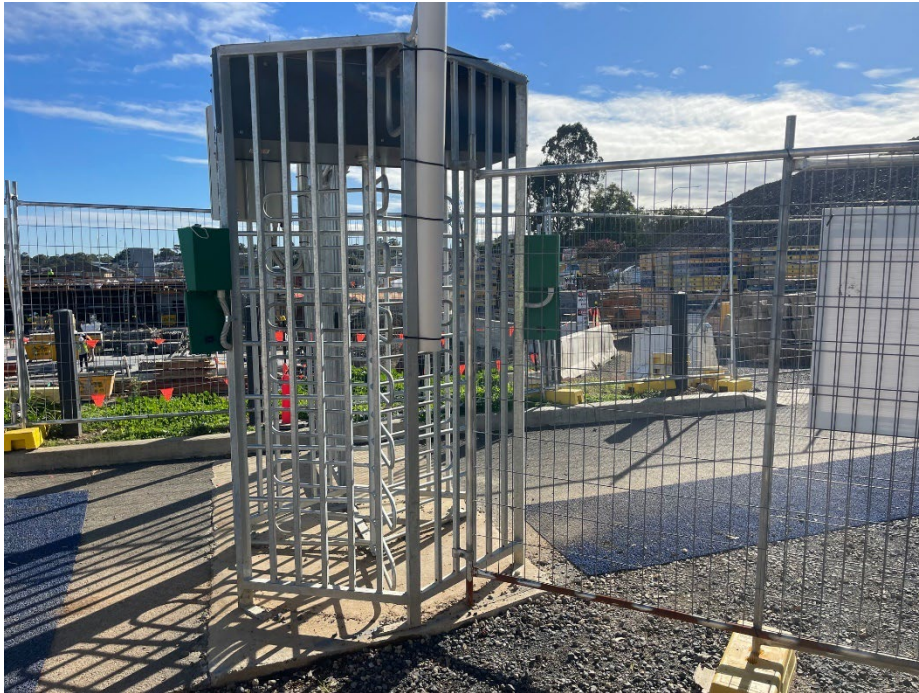
Secured turnstile to Site. Site accessible using face recognition application. Designated blue walkway throughout the site.
