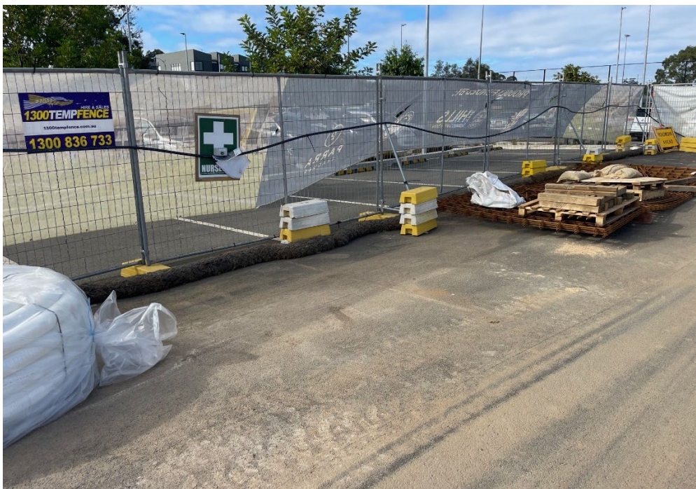
Coir logs well utilised as erosion and sediment controls in laydown hardstand areas.
