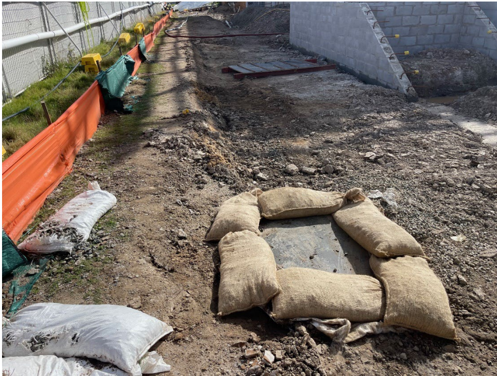
Sediment fences utilised and observed to have been replaced in certain sections as required. Pit drain also protected.
