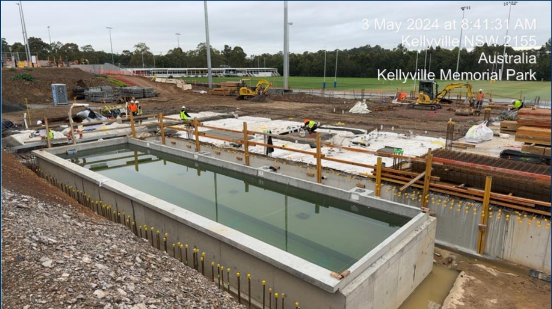
Building B – Pool water testing
